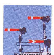
Railway Signalling & Telecom Equipment
